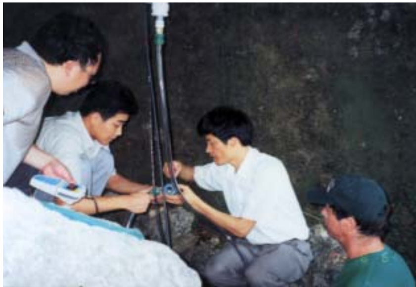
Dr. Chris Groves, Co-leader of IGCP 448 from WKU, USA, and Director of Hoffman Environmental Inst. is working with Chinese Colleagues to install data-log facilities at the Karst Dynamics Field Experimental Site in Guilin.
